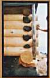
Close-up of a wooden log with a metal nail or fastener.
